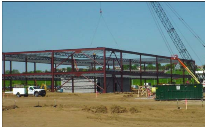
Construction is underway on PayPal's 125,000 sq. ft. expansion in the Southport East development.
